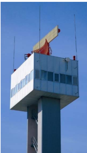
A typical antenna array: a parabolic antenna for the primary radar beneath a linear dipole array for the secondary radar. Both antennas rotate together.
