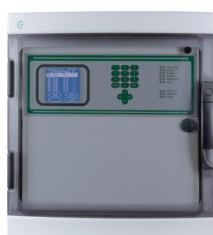
CONTROL PANEL (MULTISCAN++S1)
