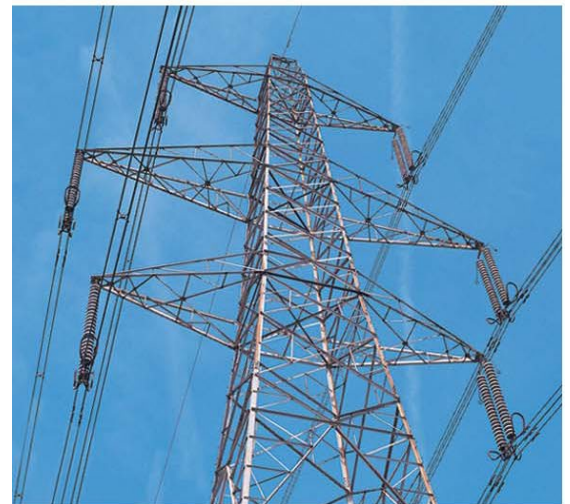
... where electrical energy is distributed
