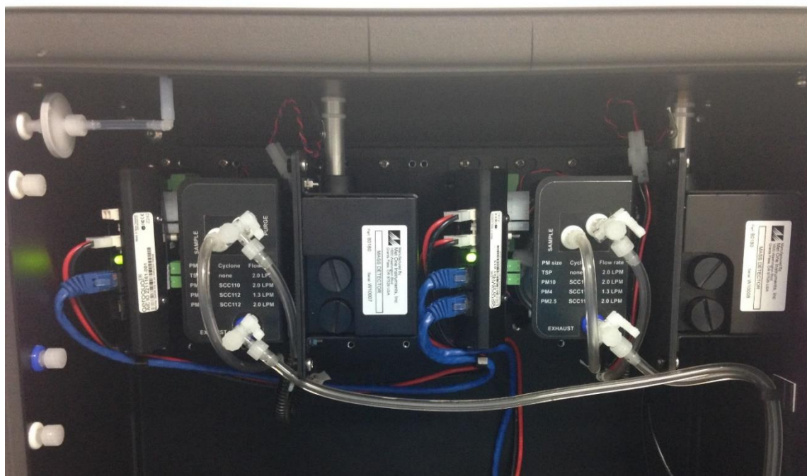
Figure 0-11 Two Particle Monitors can be installed in an AQM 65, each Particle Monitor will have three modules each
